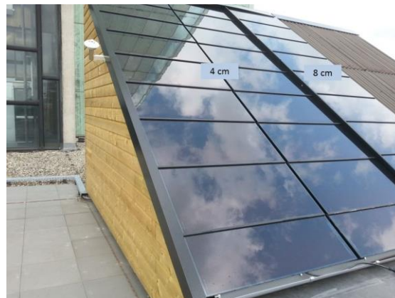
Figure 1: A dummy house with a typical Dutch attic. Three rows are used for experiments with a new BIPV-product that is combining thermal insulation and CdTe PV-panels. The insets shows the air gap depth, which is varied between 4 and 8 cm to investigate thermal effects.
