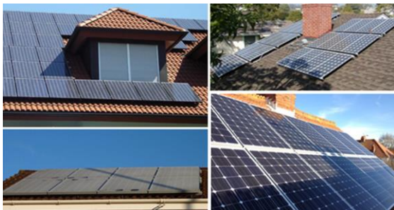
Figure 1: Light obstruction on rooftop PV systems
